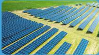
Solar Cell 2 MVA
