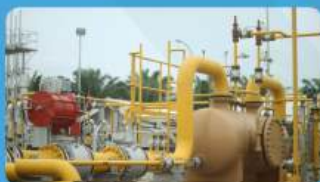
Natural Gas Pipeline 75 MMSCFD
