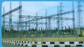
Electricity 150 KV/ 60 MVA
