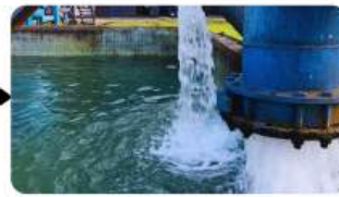
Water Treatment Plant 250 m 3 / hour
