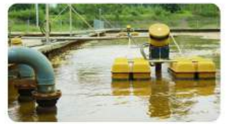
Waste Water Treatment Plant 250 m 3 / hour
